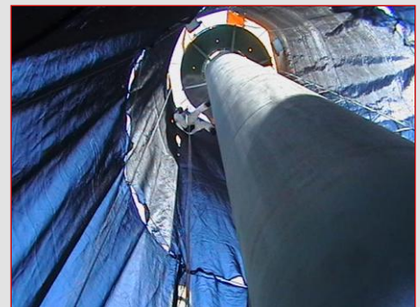
This photo above shows one of our containment solutions for a vertical stack that NZIA sandblasted and painted during a 3 day shutdown
